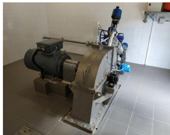
Turbine of the micro-hydro power plant
